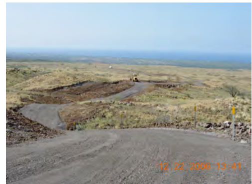
An emergency access road leading from Waikoloa Village to Queen Kaahumanu Highway was recently built to provide additional egress during wildfire emergencies.
