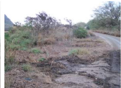
Road dip with stream debris makes for difficult access on road to Polihale
