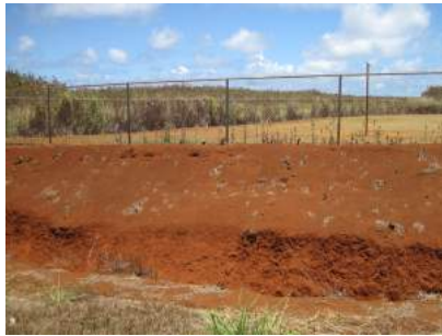
King Kaumuali'i Elementary School with eroding slope
