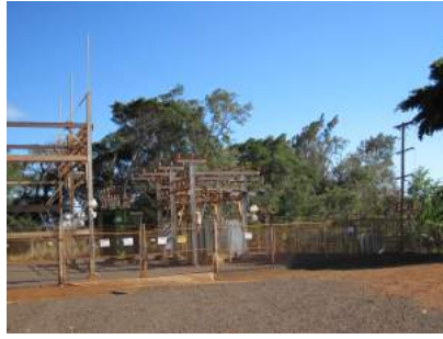
Overgrown fuels next to power generator
