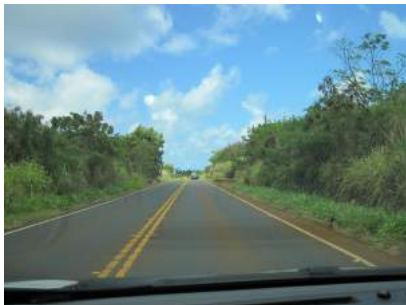
No shoulders along Olohena Road
