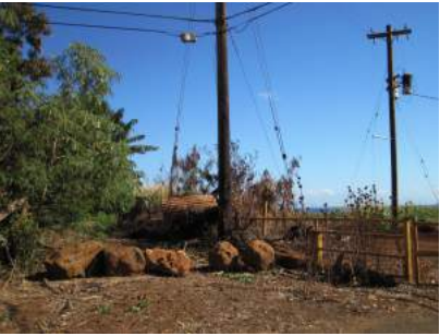
Charred vegetation under powerline at end of the street
