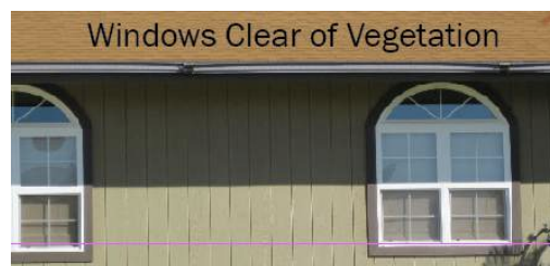
Figure 10. Keep windows free of vegetation to reduce likelihood of heat-caused breakage that lets embers into your home.
