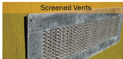
Figure 9. Covering vents with 1/8-inch or smaller metal mesh blocks embers from entering a home or structure.
