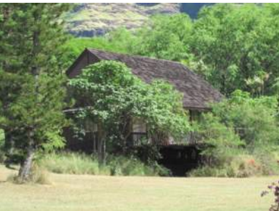
Mākaha Valley Country Club structure with shake roof and lack of defensible space
