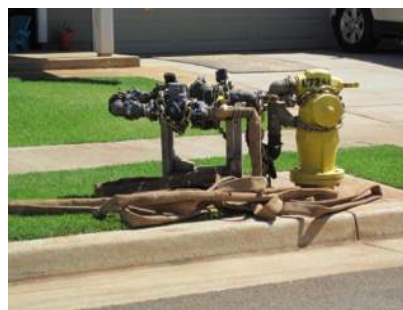
Fire hydrant and hose on Kekahili Street
