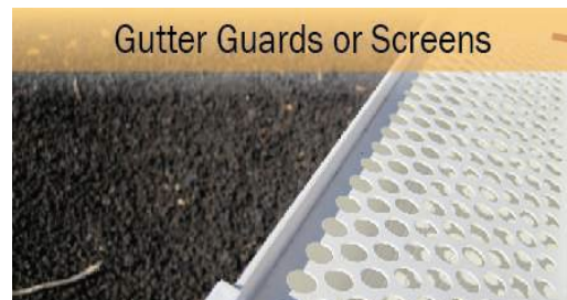
Figure 15. Rain gutters should have screens to keep leaf debris from accumulating. Maintain gutters to keep them clear and clean.
