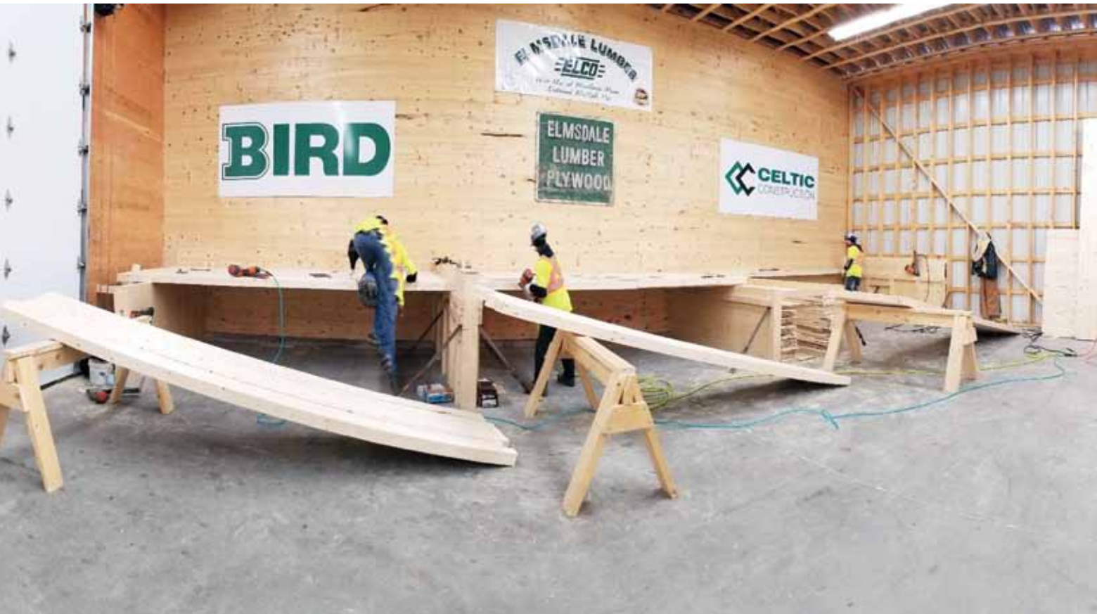
A temporary workshop set up at Elmsdale Lumber for manufacturing nail-laminated timber (NLT) panels to be used in the new East Hants Aquatic Centre.
