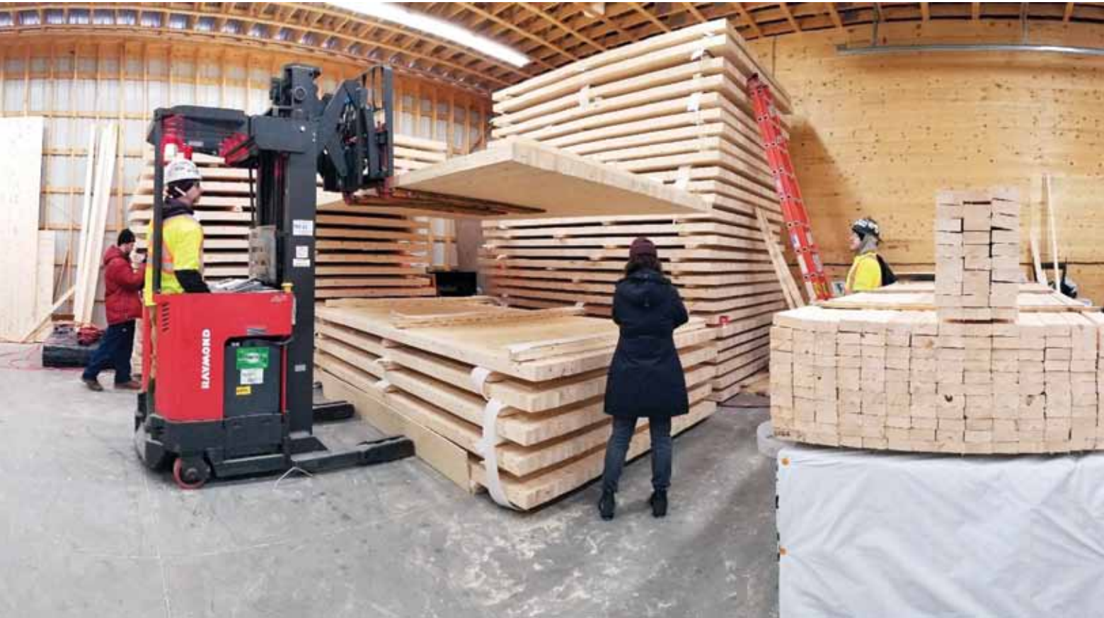
Swimming Pool Aquatic Centre, a $19 million project being built just down the road by Bird Construction.
