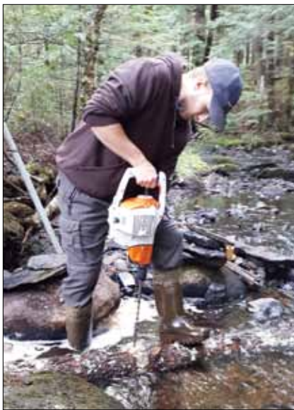
Sam Reeves, watershed and agricultural projects coordinator with Bluenose Coastal Action Foundation, demonstrating the installation of in-stream habitat restoration structures in Silver Mill Brook, which passes through the Veinotte farm and woodlot.
