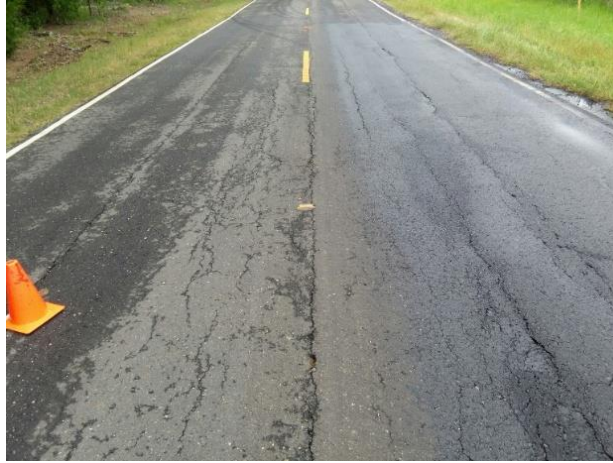
Figure 4 Longitudinal cracks in roads in Caddo Parish, LA
