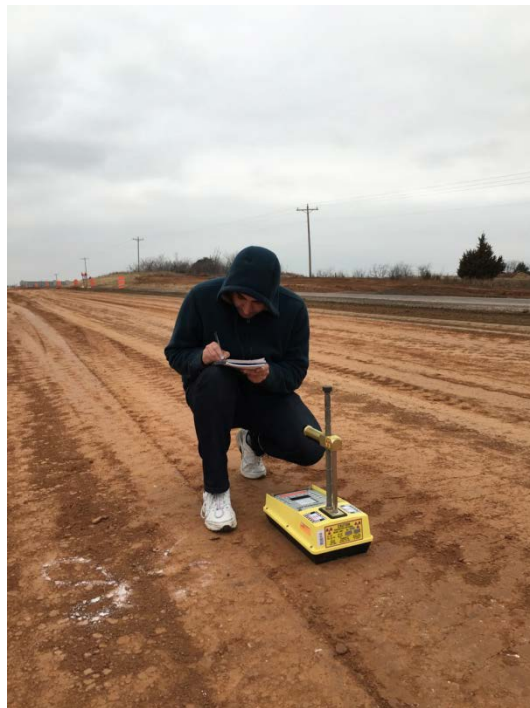
Figure 12. Recording density and moisture content on compacted subgrade using a Nuclear Density Gauge
