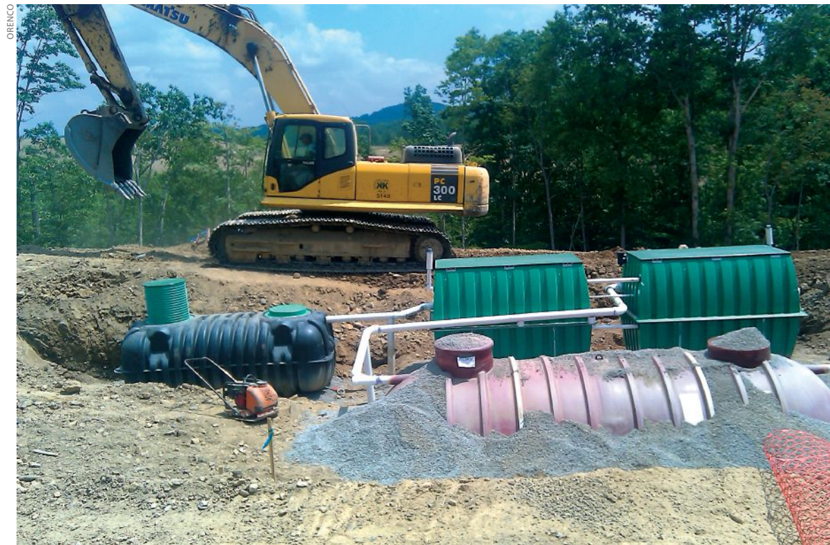
Installation of the onsite wastewater treatment and reuse system by Orenco Systems at the Summit Bechtel Reserve—Boy Scouts of America Jamboree site
