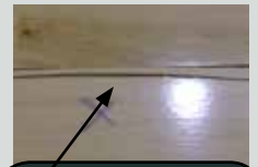
Split board due to side bonding
