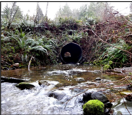
Before: Five foot diameter undersized culvert on Field Creek impeding fish passage.
