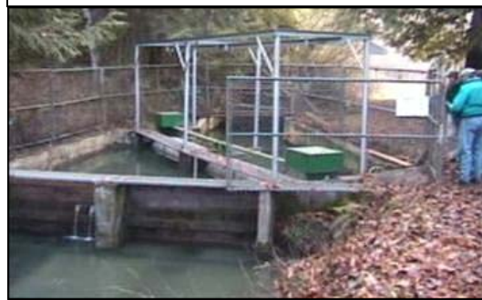
Exhibit 2-34 Fish Screens on Independent Canal Diversion
