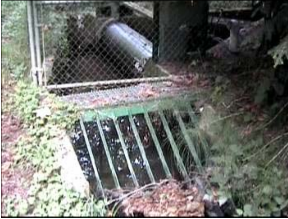
Exhibit 2-19 Agnew Fish Screen at McDonnell Creek
