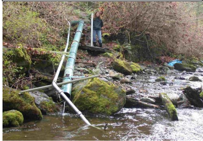
Exhibit 2-20 Agnew Fish Bypass Pipe on McDonnell Creek
