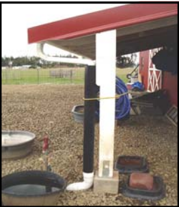
Downspout carries roof water via pipe to drywell.
