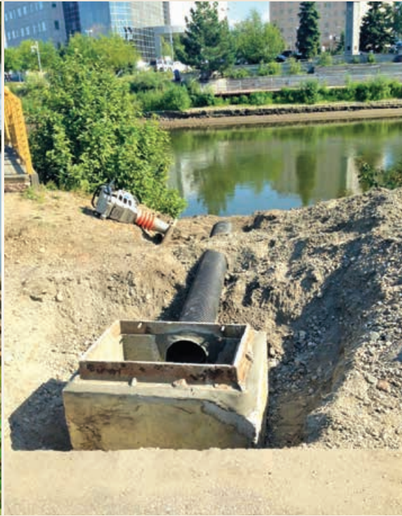
The city installed this catch basin to receive the runoff and capture some of the sediment and litter before spilling the water down the newly vegetated bank.
