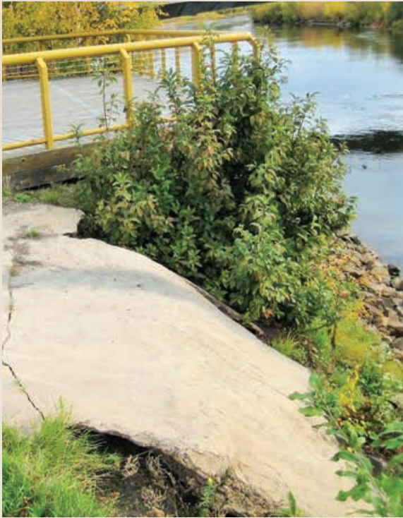
Polluted runoff from the 21,000 square-foot parking lot at Gordon Wear Park drained directly into the river via this concrete chute.
