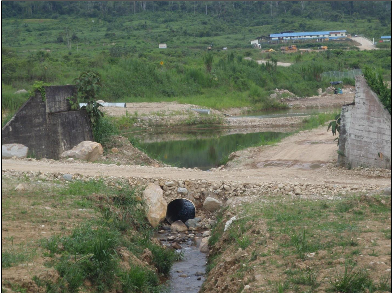
Figure 19a. The overflow from the sedimentation ponds for the Tundayme tailings management facility is discharged into a pipe and flows to the Rio Quimi (see Fig. 11). Photo taken by the author on November 6, 2018.
