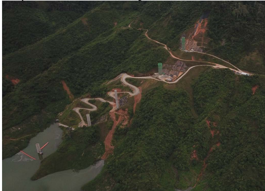
Figure 7. Decant Towers under construction. The tower in the lower left appears to be operational. Towers higher on the hillside are for future use. Late May 2022. Source: locally provided photograph.
