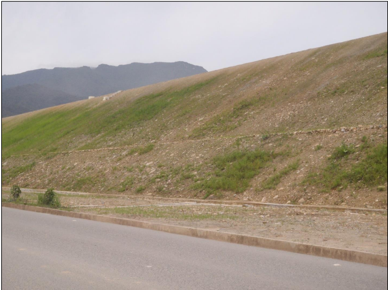
Figure 16. The starter dike for the Quimi tailings dam was built at the edge of the highway, the other side of which is the Rio Quimi (see Fig. 11). Since it is not possible to advance the dam farther in the downslope direction, the intention must be to build the entire dam using the upstream method (compare Figs. 5a-c). This is inconsistent with the design evaluated by Knight-Pièsold (2007) and both Environmental Impact Studies (Walsh Scientists and Engineers, 2010b; Cardno, 2014a), which included the centerline construction method for the Quimi tailings dam. Tailings dams built by the upstream method are more susceptible to failure from both earthquakes and floods. Due to the impossibility of installing impermeable layers (see Figs. 5a-c, 8), their higher water content also makes them more susceptible to failure due to internal erosion, static liquefaction and foundation failure. Photo taken by the author on November 6, 2018.
