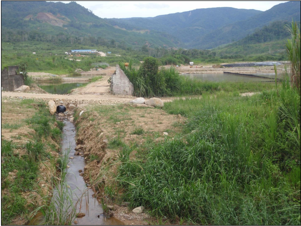
Figure 19c. The gray color of the discharge from the sedimentation pond demonstrates that the sedimentation ponds are not working (Quishpe Lozano et al., 2018). Photo taken by the author on November 6, 2018.
