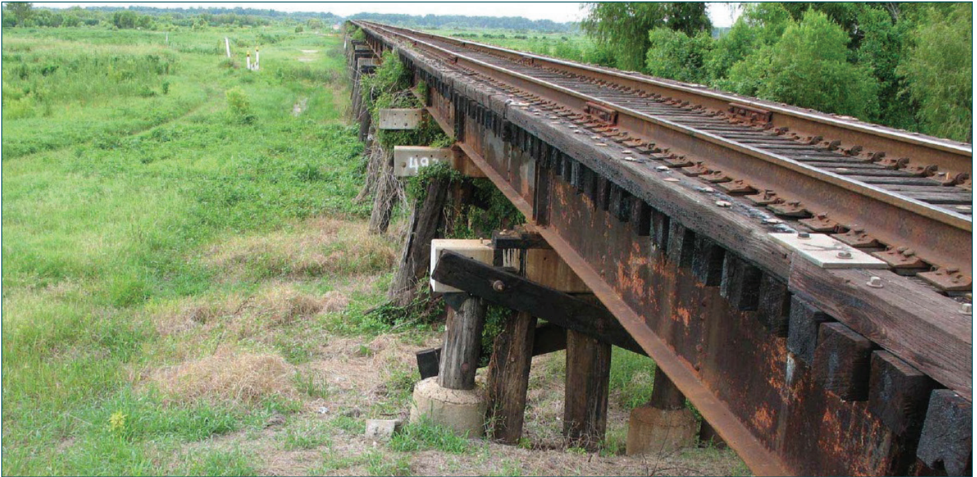
▲ Figure 8: The single track Bonnet Carré Spillway Bridge, with its 10 mph speed limit, is a major impediment to the growth of the freight traffic on the rail line.
