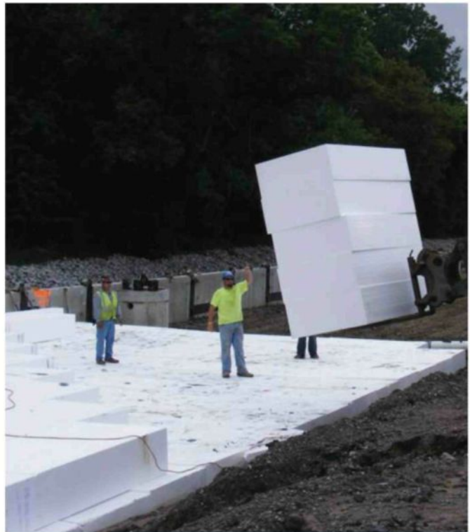
The geofoam used in the Gary, Ind., highway project is equivalent to more than 400 dump truck loads of earthen fill.
