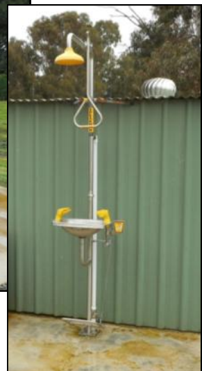
The safety wash area
