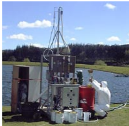
Jetflote pilot plant trials being done on location beside the oxidation ponds at Waihi.
