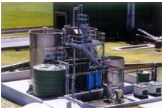
Complete industrial waste water treatment plant including IAF for solids-liquid separation.
