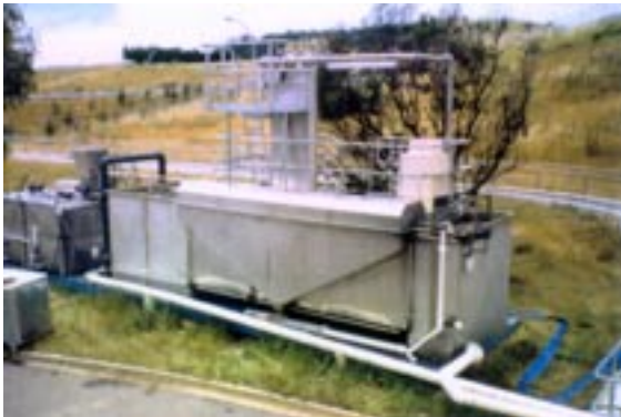
IAF at 4ML per day wastewater treatment plant.
