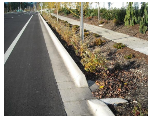
Bio-swale that conveys flows along an arterial street. Source: Nevue Ngan Associates
