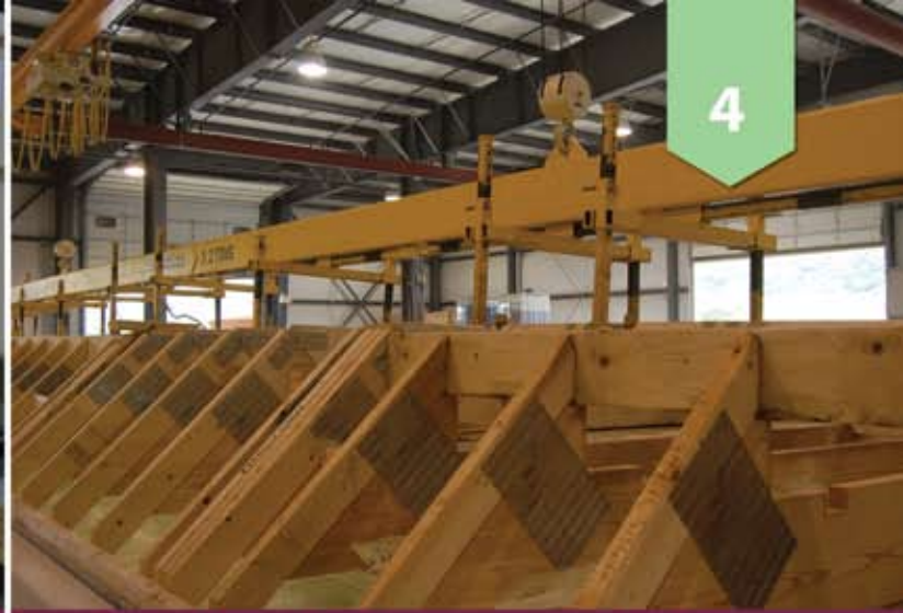
The roof is constructed with engineered roof trusses on a square and level jig, and hoisted onto the home with a 3-ton crane.
