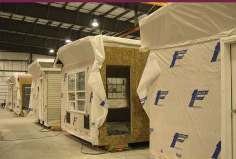
Modules move along the assembly line, completing electrical, drywall, and other finishes.
