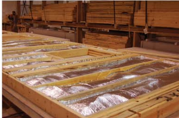
Construction of exterior wall, featuring 2"x6" wall studs, 16" on-center, with optional Energy Wall insulation package.
