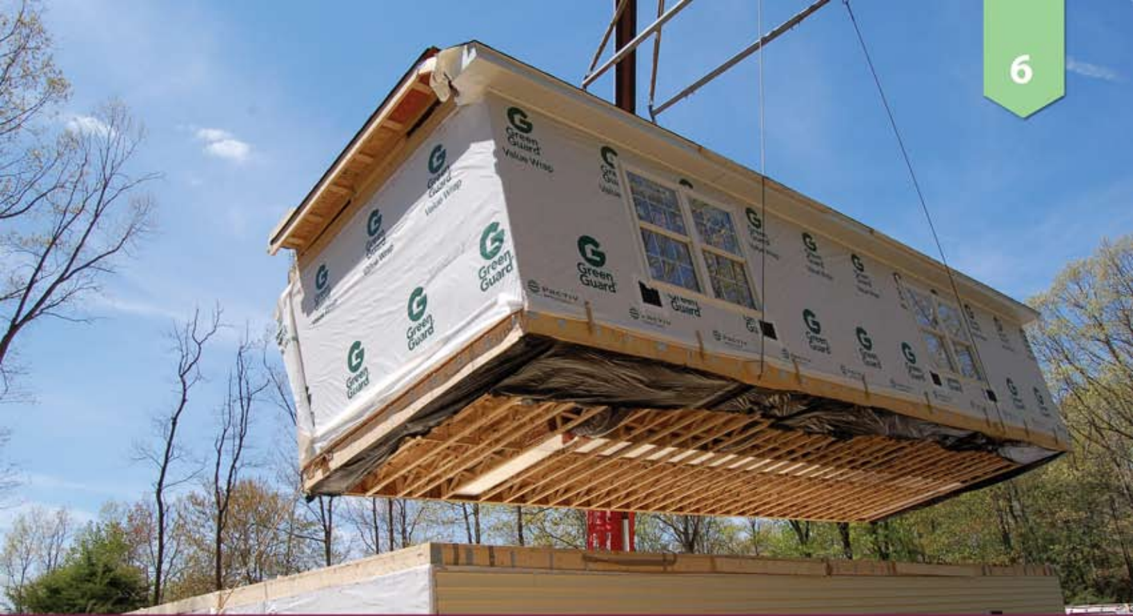
3. On the day of set, each module is lifted into place with a crane.
