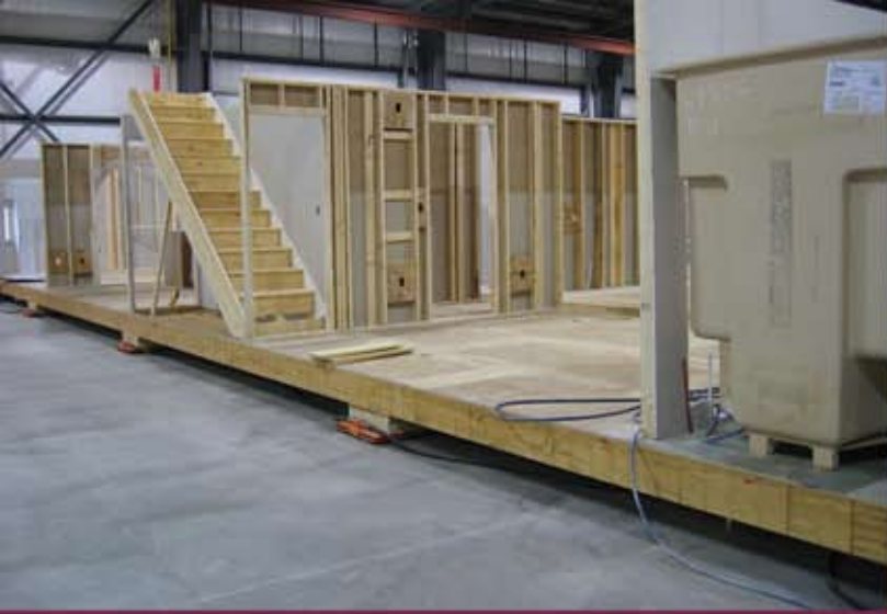
All floors, walls, and roofs are built on a laser-leveled factory floor.
