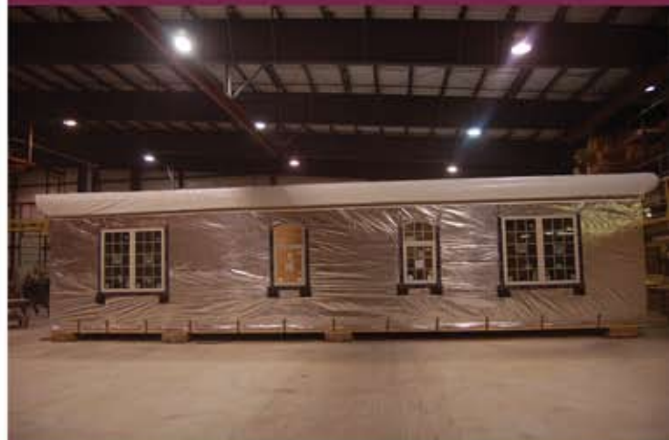
A module moves down the production line, showing exterior wall with optional Energy Wall insulation package.
