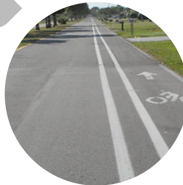
Buffered bike lane in a residential area of Cape Coral, FL. Solid white lines are used when the buffer zone is less than three feet wide. Source: NACTO
