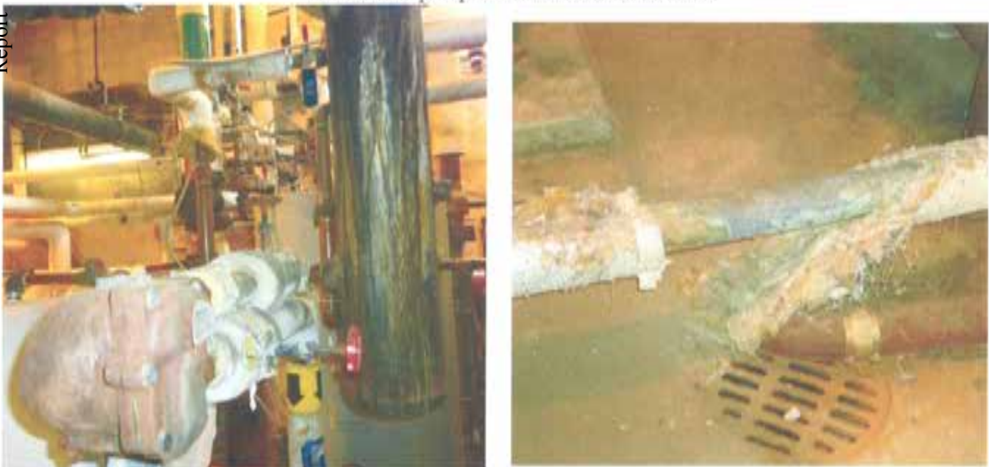
FIGURE M-13: Severely Corroded Piping & Deteriorated Insulation in Hemberger Basement
