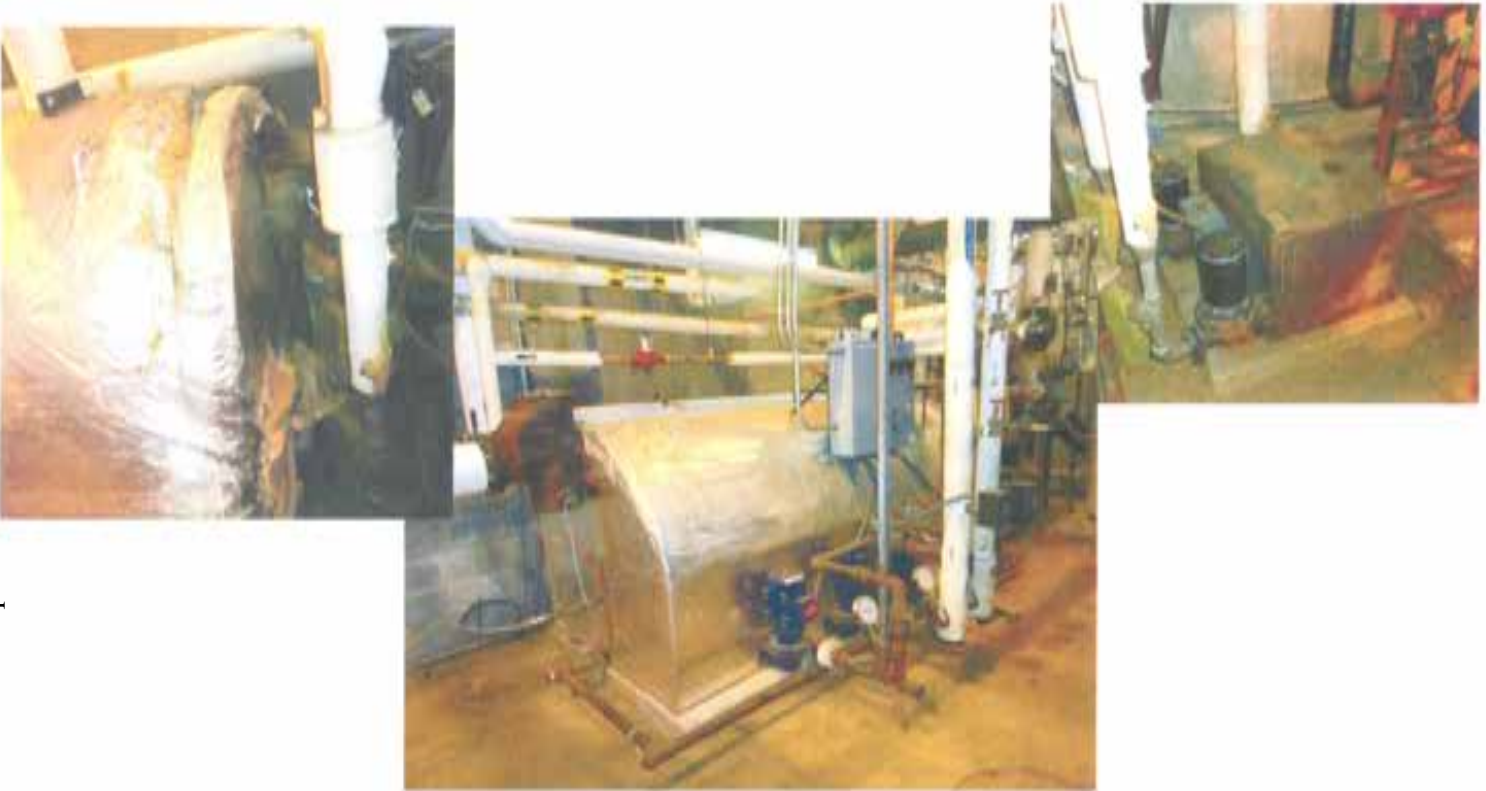
FIGURE M-12: Hemberger Tower Boiler room Boiler feed tank & close-ups of condensate pump & Insulation deterioration
