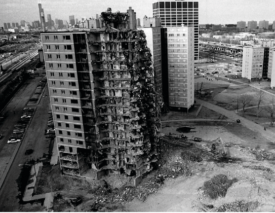
The first building to be demolished at Stateway Gardens with the downtown Chicago skyline in the background.
