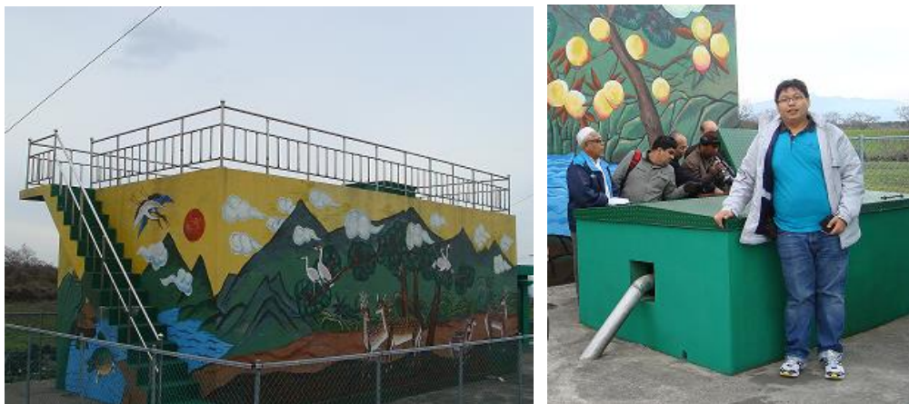
The view of storage plant and production well
