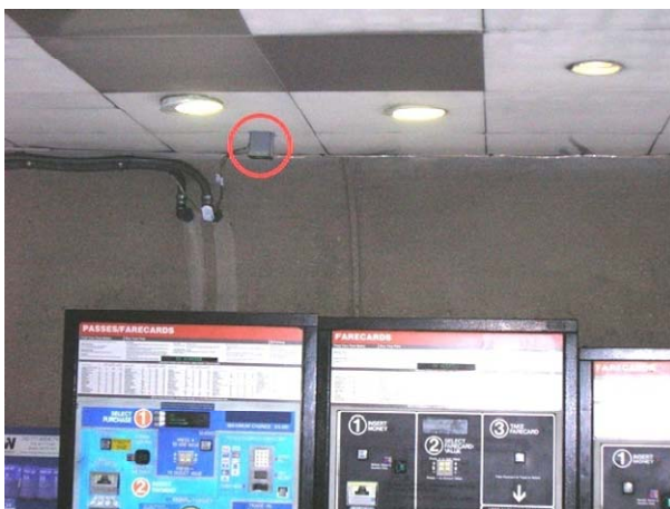
Figure 5. One of three cameras (circled) deployed in a test installation of the GammaPix technology at the Medical Center Station of the Washington, D.C., Metro system.
