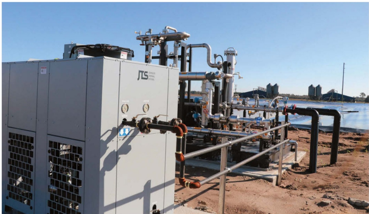
Stations next to each covered digester pre-conditions the bio-gas before going to the refinery.
