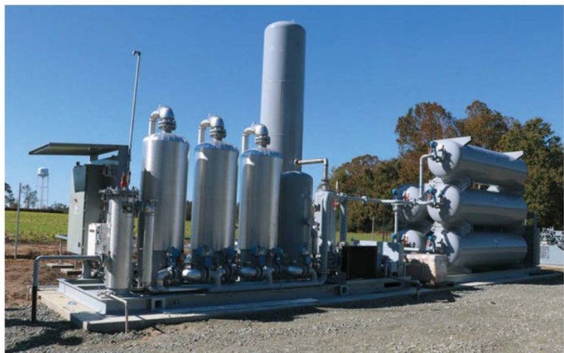
Methane goes through a multi-stage cleaning process and automated testing before being released into the pipeline.
