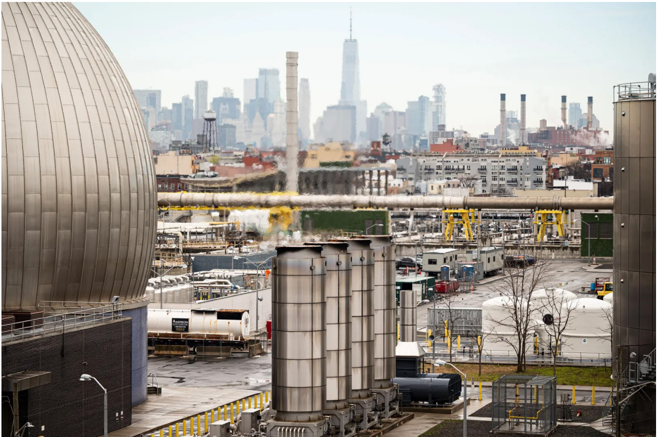
The flares at Newtown Creek (seen here) will no longer burn off unused biogas with the implementation of the innovative "gas-to-grid" model.
