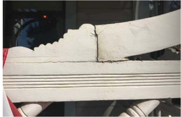
Wood decay and separations at porch trim. (ARG, 2016)
