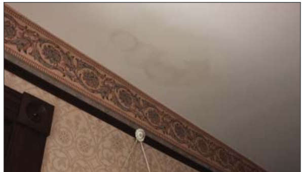
Stains at dining room ceiling from previous leak. (ARG, 2016)
