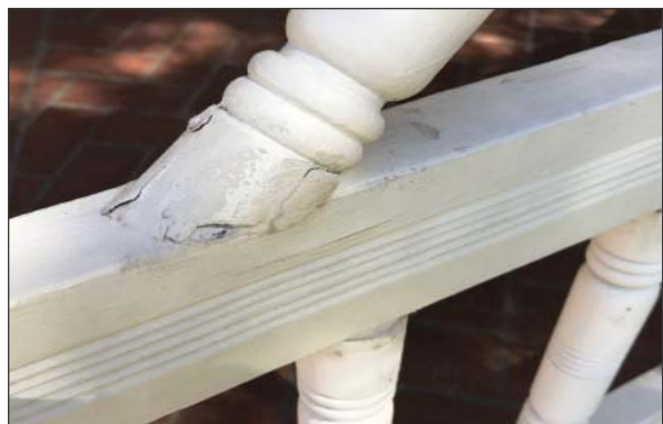
Deteriorated/ spalling prior wood fill repairs. (ARG, 2016)
