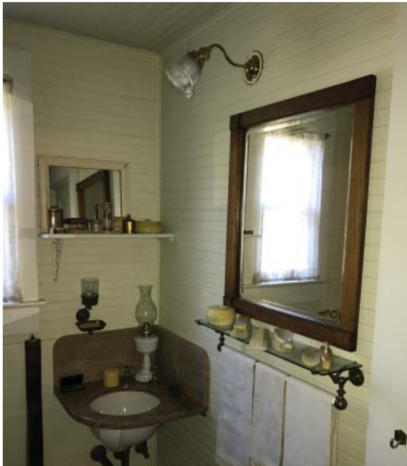
Painted bead board paneling at walls and ceiling of second floor bathroom. (ARG, 2016)
