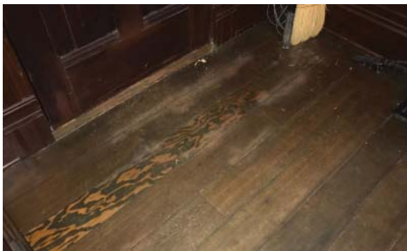
Abrasion/ wear of stained finish at kitchen entrance. Also note prior repair with mismatched wood. (ARG, 2016)
