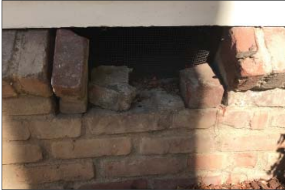
Loose brick units at crawl space vent, south elevation. (ARG, 2016)
