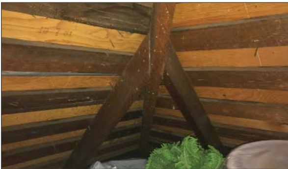
Structural roof framing at attic storage area. Also note spaced roof sheathing boards and plywood sheathing overlay. (ARG, 2016)
