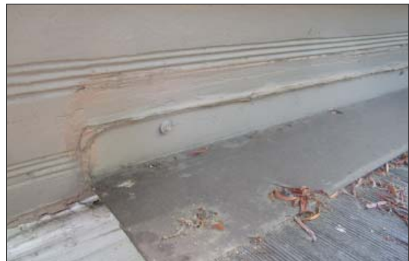
Typical painted sheet metal wall flashing. Note screw fasteners and sealant joint. (ARG, 2016)
