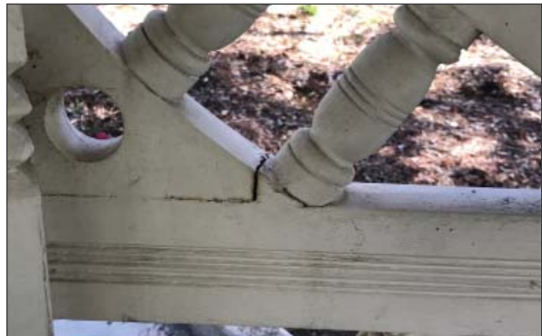
Separations and loose components, soiling and decay at railing. (ARG, 2016)
