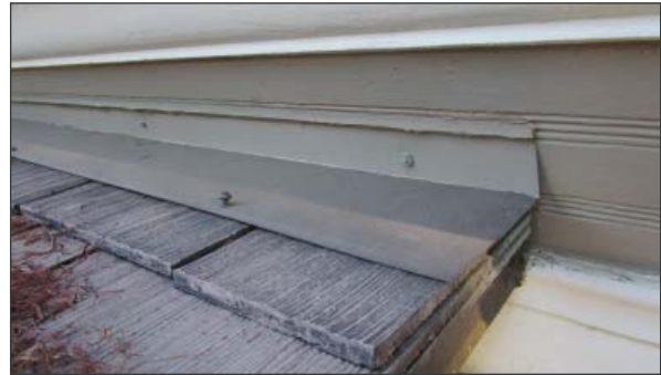
Loose screw fasteners at metal flashing. (ARG, 2016)
