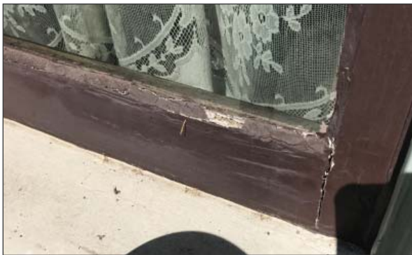
Deteriorated putty and separation in sash at south elevation bay windows. (ARG, 2016)
