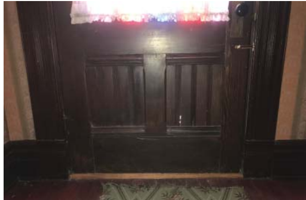
Daylight seen through separations in recessed bead board panels at front door. (ARG, 2016)
