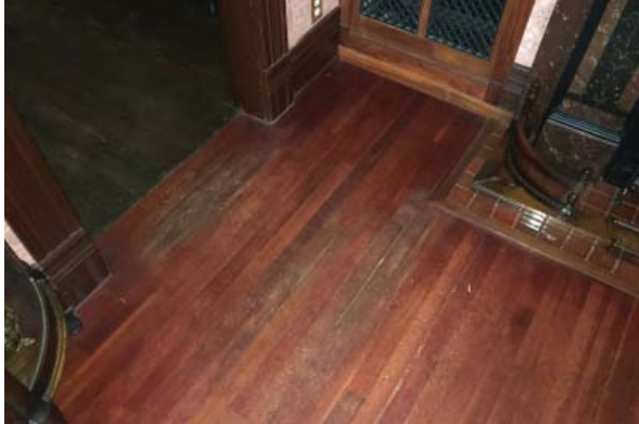
Burgundy-stained fir floor at dining room, and green-stained pine floor at kitchen beyond (top left). Also note abrasion/wear from foot traffic. (ARG, 2016)
