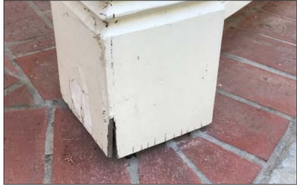
Decay, splitting, and peeling paint at base of column. (ARG, 2016)
