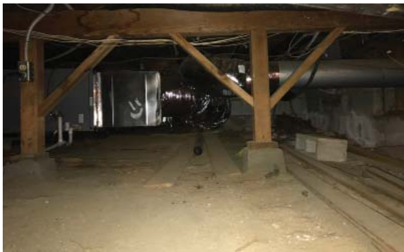
Crawl space and concrete pier footings. Note misc. lumber at grade. (ARG, 2016)
