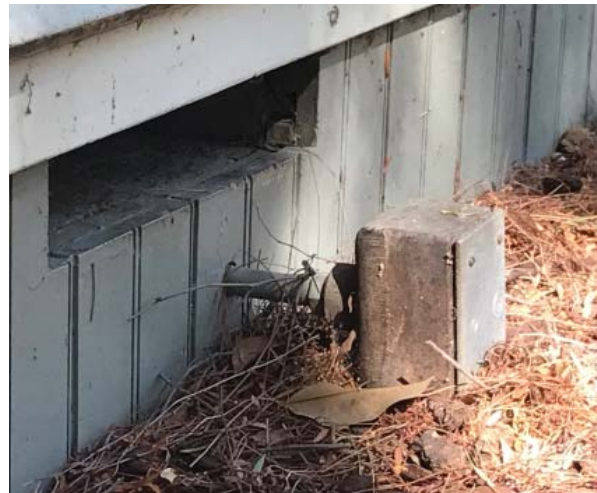
Outdoor junction box at northeast porch, partially buried by debris. (ARG, 2016)
