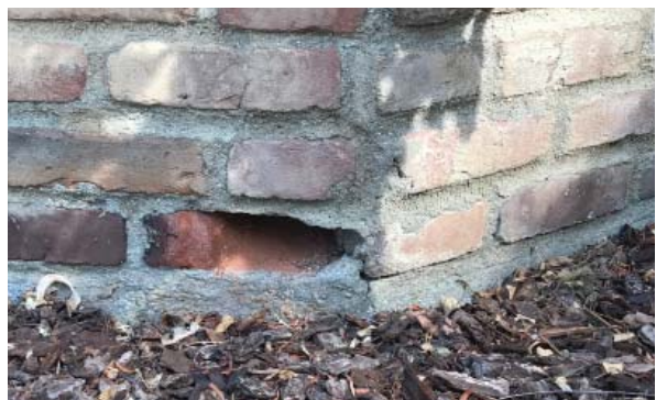
Eroded brick unit at foundation wall, south elevation. (ARG, 2016)
