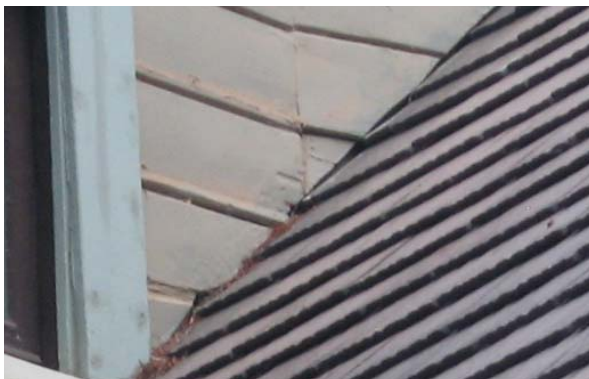
Wood decay and splits at base of shingles near roof surface. (ARG, 2016)
