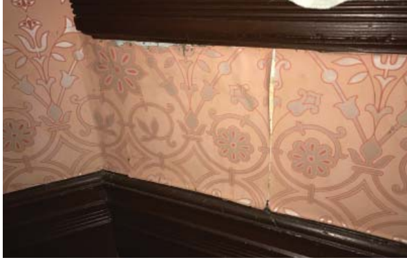
Tears and lifting of seams at dining room wallpaper. (ARG, 2016)
