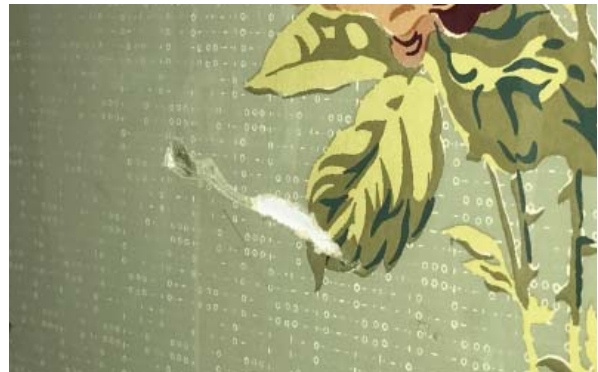
Gouge at stair hall wallpaper. (ARG, 2016)
