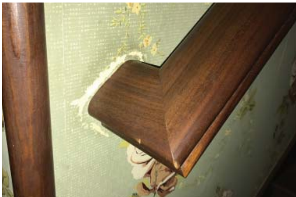
Wallpaper stains and wear/loss at stair handrail. (ARG, 2016)
