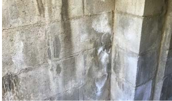
Efflorescence and staining at CMU walls of basement stair. (ARG, 2016)
