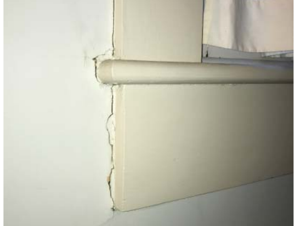
Separations between wall and trim at window casing in child's bedroom, second floor. (ARG, 2016)
