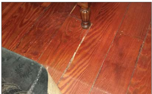
Split at floor board below chest of drawers in master bedroom. Also note stain color difference below carpet. (ARG, 2016)
