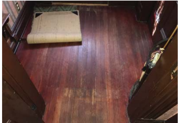
Abrasion/ wear of stained finish at entry vestibule floor. (ARG, 2016)
