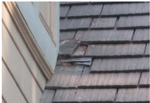
Cracked and loose tiles at south elevation adjacent to tower. (ARG, 2016)
