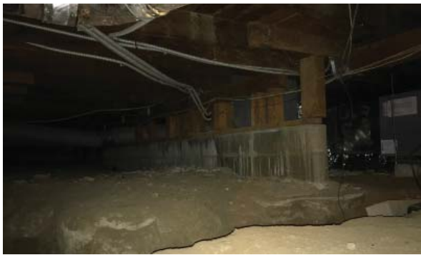
Crawl space and concrete stem wall foundations. Note water staining at stem wall. (ARG, 2016)
