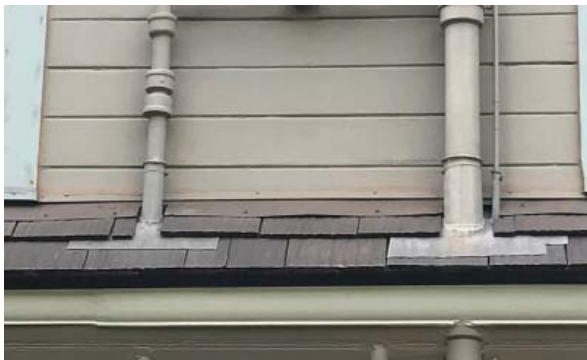
Sheet metal flashing at dormers. Note sealant at wood siding, evidence of prior flashing installation. (ARG, 2016)
