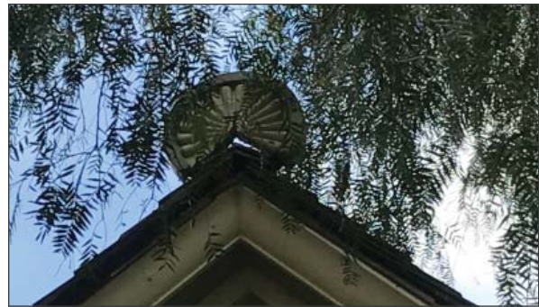
Wood decay and ill-fitting, possibly loose, spoked wheel trim at east gable. (ARG, 2016)
