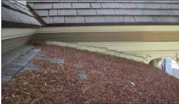
Heavy debris accumulation at southwest porch. (ARG, 2016)
