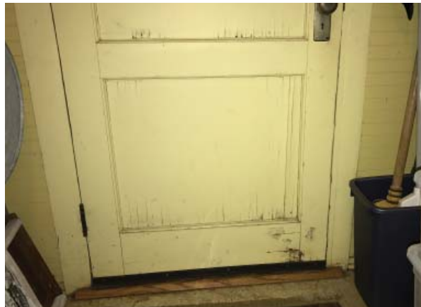
Multiple splits and wood decay at door to west enclosed porch. (ARG, 2016)
