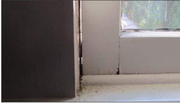
Minor splits at window sash. Also note daylight between sash and frame. (ARG, 2016)
