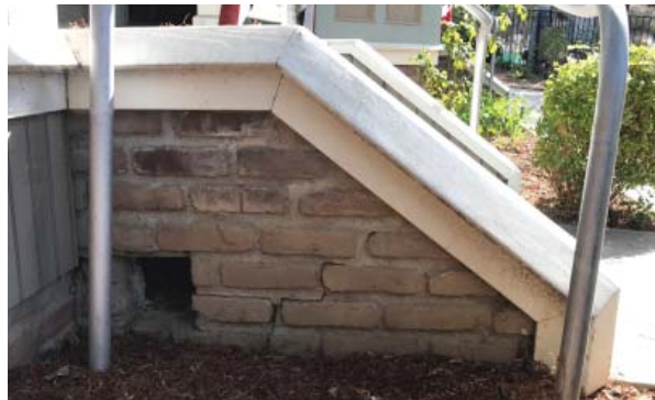
Cracking through mortar joints at brick stair wall, south elevation. (ARG, 2016)
