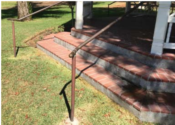
Quarry tile steps, stucco parge coating at risers, and copper tube handrails. (ARG, 2016)
