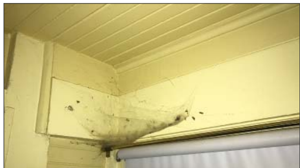
Soiling and cobwebs at utility room entrance. (ARG, 2016)
