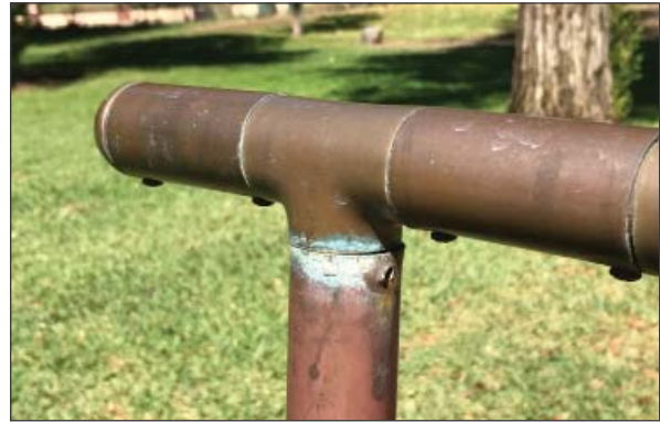
Oxidation at copper tubing. (ARG, 2016)
