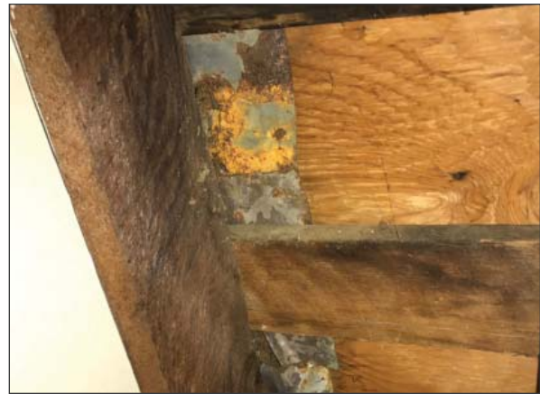
Corroded sheet metal flashing, visible from attic storage area. (ARG, 2016)
