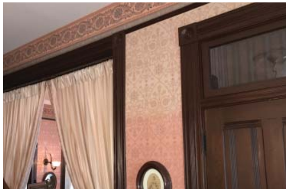
Color shift/ fade at dining room wallpaper. (ARG, 2016)
