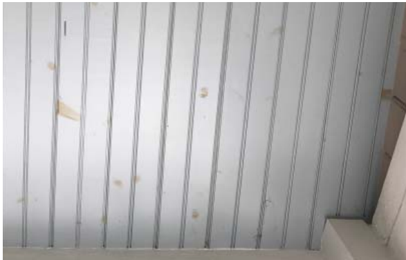
Stains at southwest porch ceiling. (ARG, 2016)
