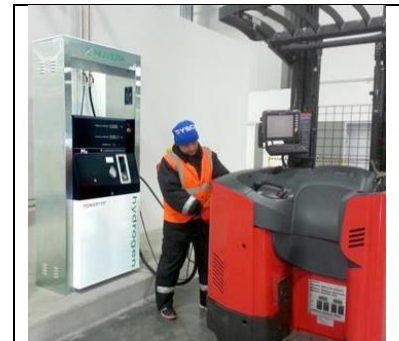
Hydrogen Dispenser - Sysco Facility
