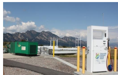
Wind-to-hydrogen facility at NREL
