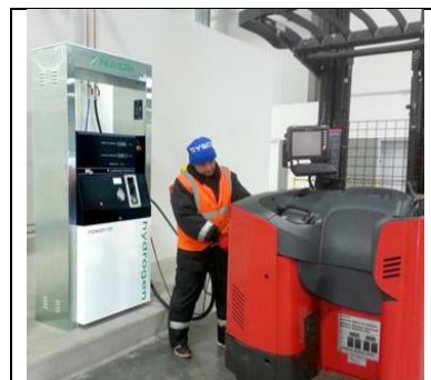
Hydrogen Dispenser - Sysco Facility
