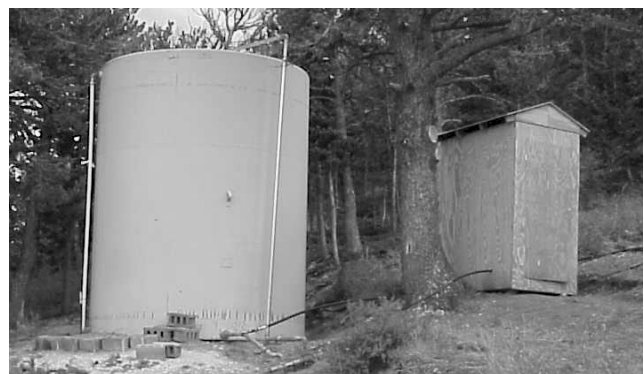
New Pump House Built by Ray Raymond, and Modifications to Tank Piping to Improve Chlorine Mixing
