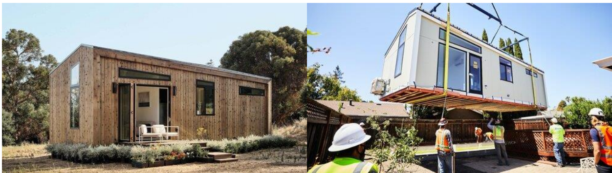
Left: Prefabricated ADU displayed in the environment it was designed for. Right: The same ADU being forced into the messy environment that characterizes backyards and alleys.
