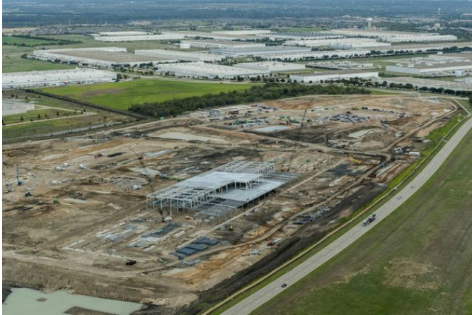
Construction of Facebook’s newest data center is underway in North Fort Worth.
