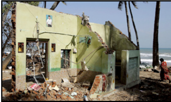
A woman on Wednesday walks past a house destroyed by tsunami at Devanahpattinam, in the southern Indian state of Tamil Nadu.
