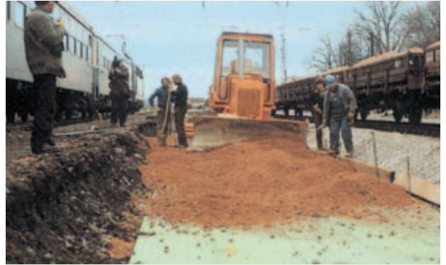
Fig. 8: Frost protection for track beds with Styrodur C featuring high compressive strength.
