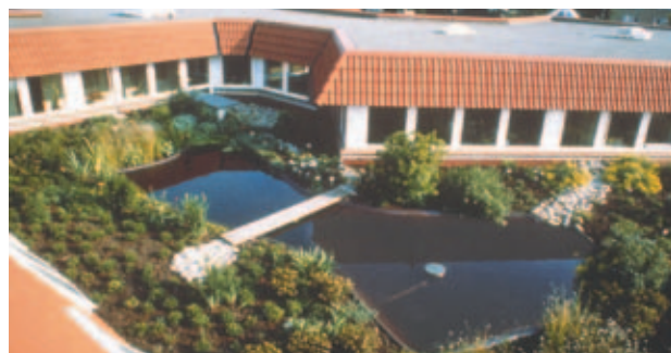
Fig. 6: Vegetated, accessible roof terrace with irrigation system of ponds on an inverted roof construction with full gravel drainage course.
