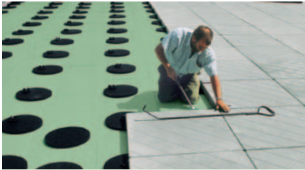
Fig. 7: Parking roof with concrete slab pavement on inverted roof with Styrodur® C.
