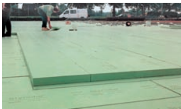
Fig. 29: Installation of Styrodur® C boards during the construction of a passive house.
