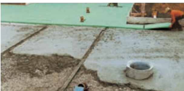
Fig. 18: Blinding layer made from lean concrete for the installation of ground insulation.
