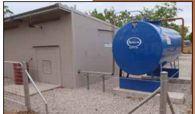
The fuel tank is regularly topped up to ensure adequate diesel is available
