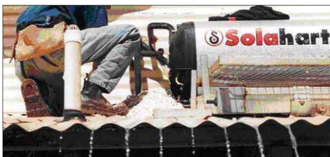
Figure 3: A maintenance worker cleans scale from a solar hot water system. Gutters should be blocked so that the scale does not flush into the rainwater tank.
