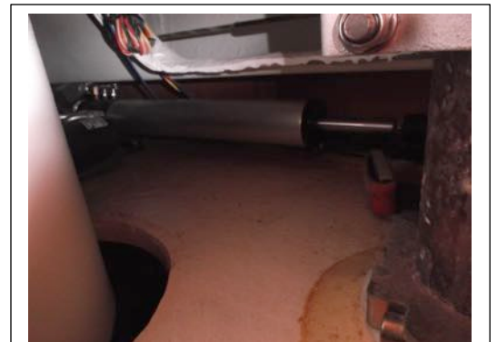
Leaking auto pilot ram
