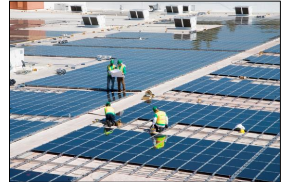
Workers install solar panels on the roof of a Walmart in Mountain View, California.
