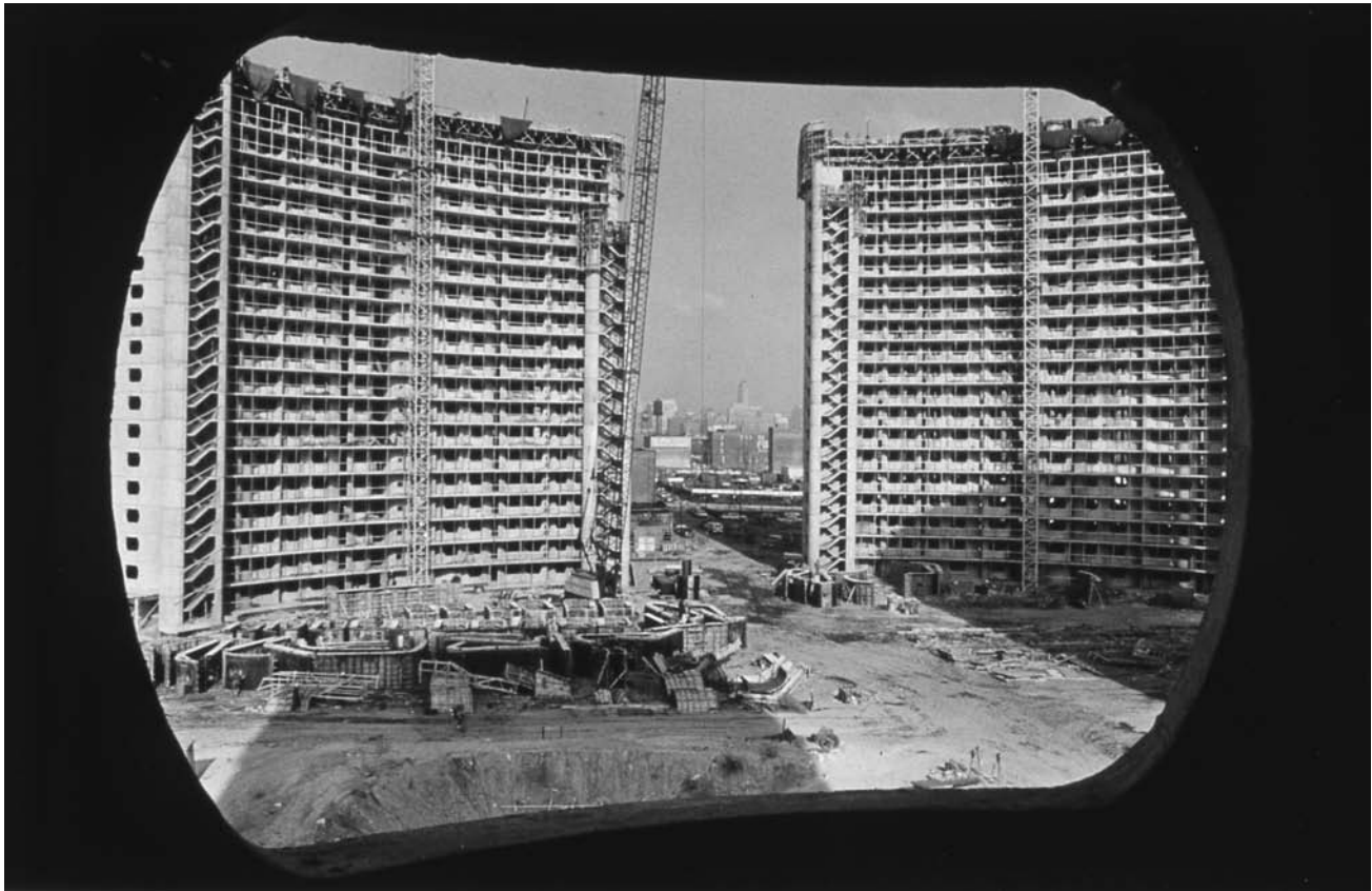
Figure 16 Bertrand Goldberg Associates, Raymond Hilliard Homes, Chicago, ca. 1966, construction view from an elderly housing unit (photo by Orlando Cabanban; Bertrand Goldberg Archive, Ryerson and Burnham Libraries, Art Institute of Chicago).
