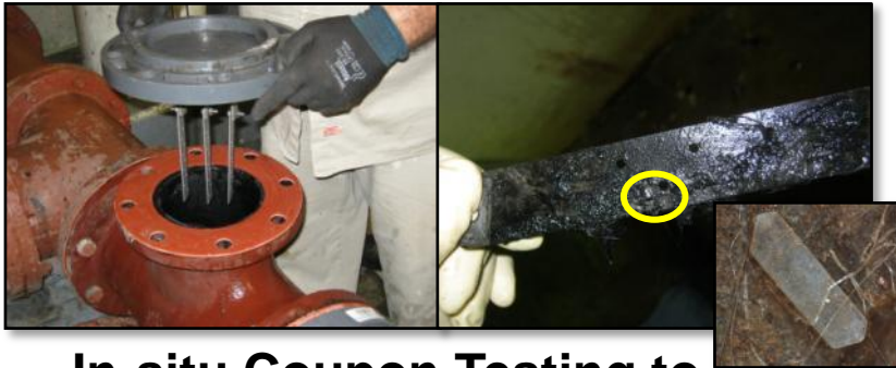
In-situ Coupon Testing to Determine Degree of Struvite Formation and Confirm Theoretical Ferric Dose
