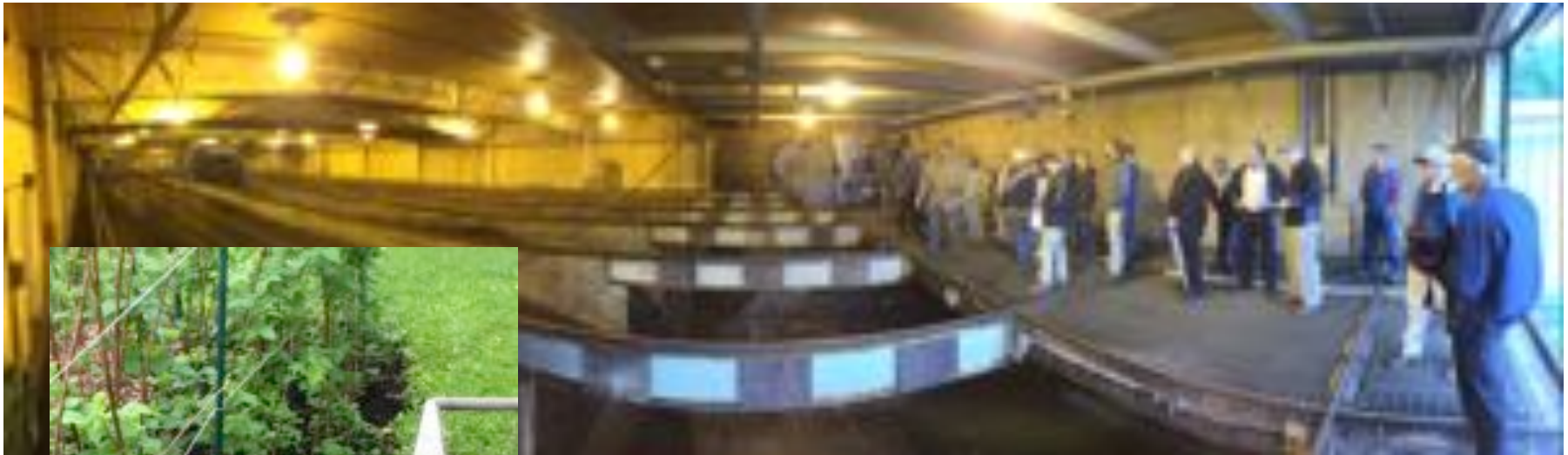
Lewiston-Auburn WPCA biosolids composting facility
