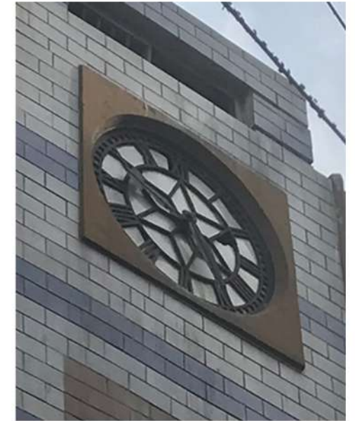
The clock is broken and not functioning but all of the outer parts still exist and shows there is potential to be fixed.
