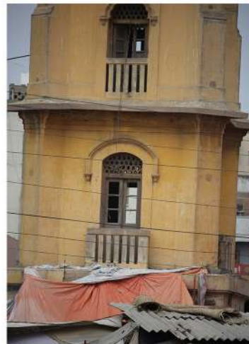
The glass on the windows of the tower are missing while the shutters are worn and broken.
