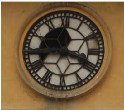
A close up of one of the four faces of the clock. The hands are intact while parts of the dial are broken.
