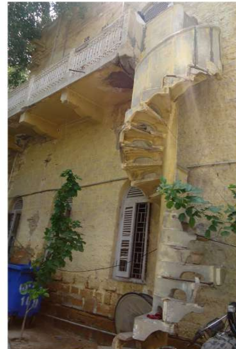
The stairs that lead up to the residential area on the second floor of the building.
