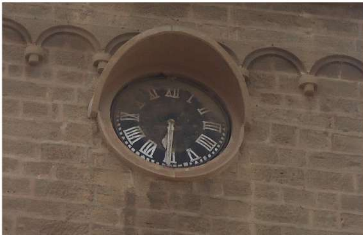
A close up of the tower shows the neglected state of the non-functioning clock as thick layers of dust have visibly piled up onto it.
