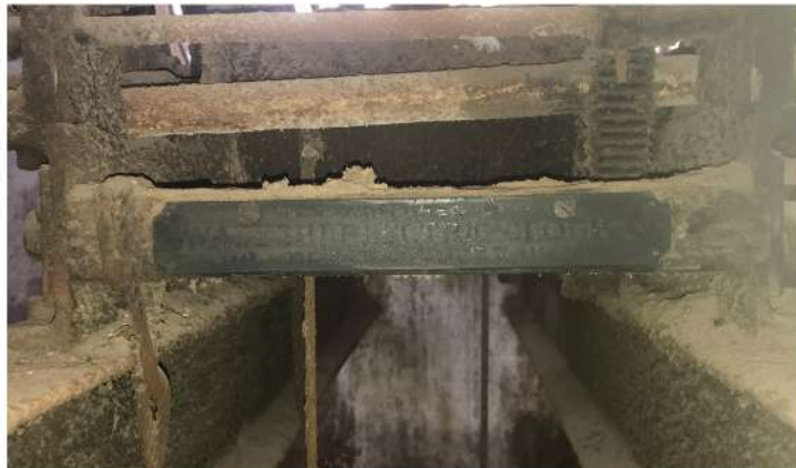
The name of the manufacturer engraved on the machine of the Poona Bhai clock tower. The engraving reads 'Swadeshi Electric Clock Company, Bombay No.7.'
