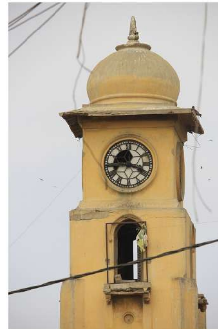
A close up of the dislodged shutters and the broken window sill of the tower.
