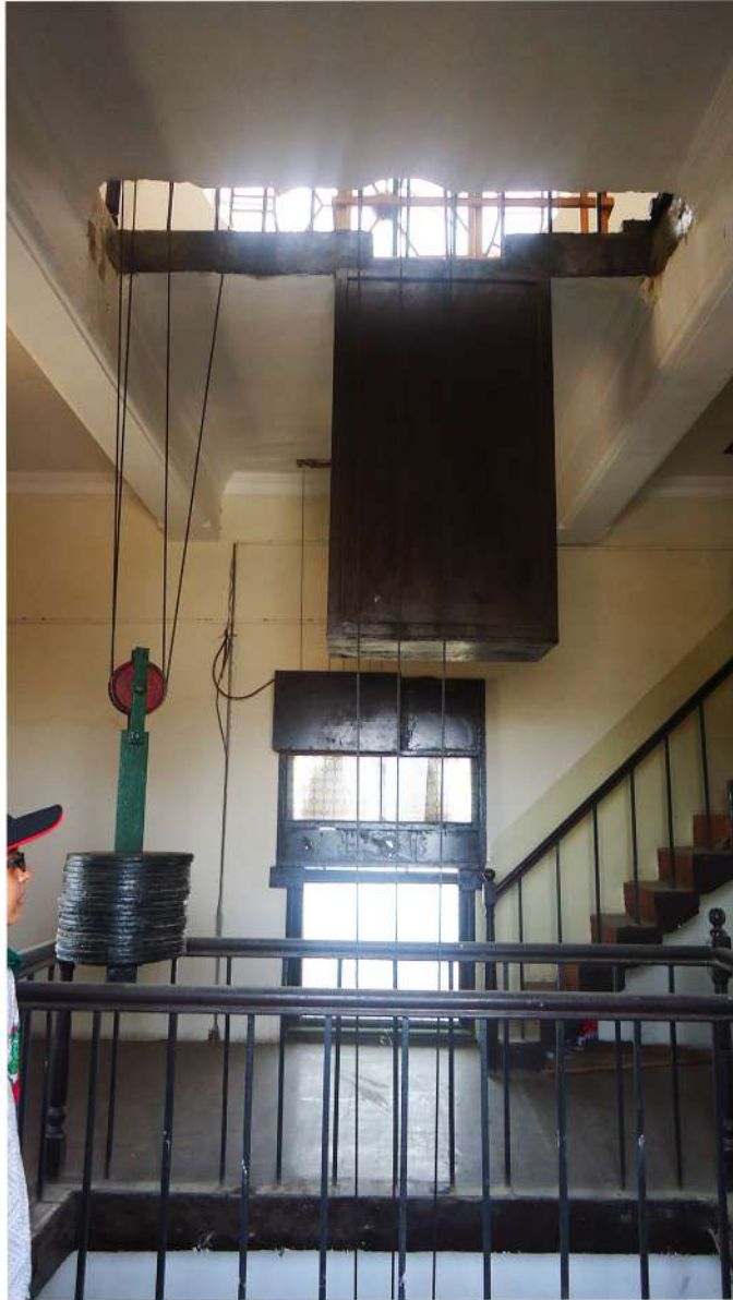
A view of the inside of the clock tower from the first floor with the exposed mechanics of the clock and bell.
