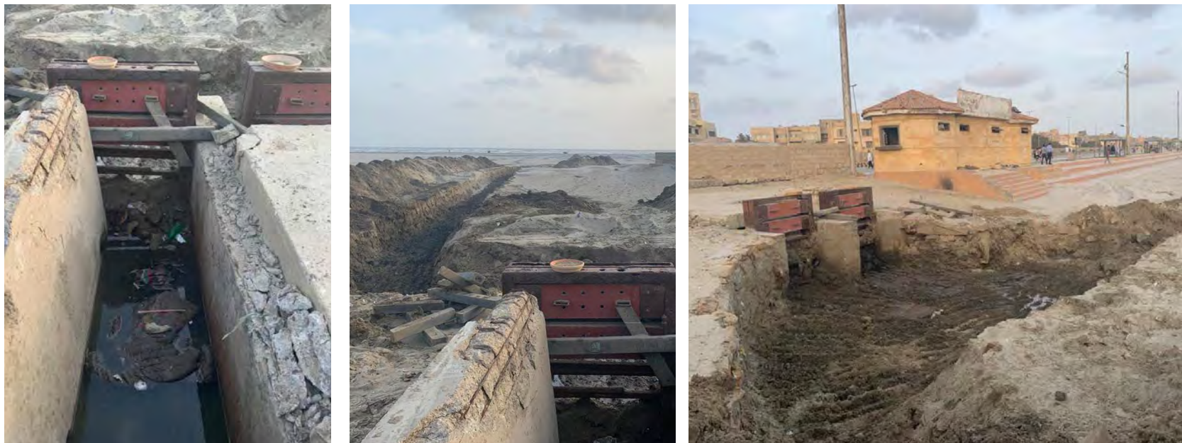
Photographic Examples of Sewage Paths along the Edge from Site Visit
