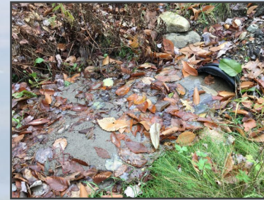
A clogged culvert in the watershed
