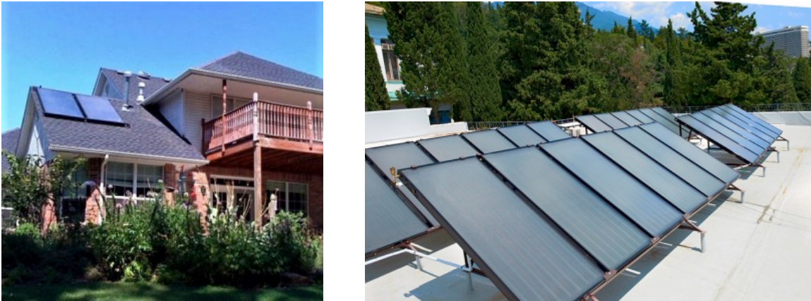
Figure 10. Examples of installed solar thermal panels in residential (left ) and commercial or multifamily (right).
