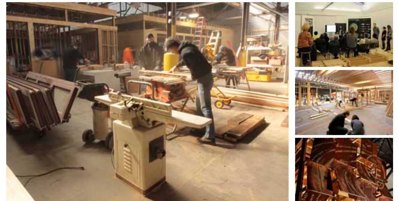
this page, clockwise from top: exploded perspective drawing; design review photo; construction framing; entry marquee; exterior cladding construction. opposite: View from workshop featuring reused hollow-core door entry canopy, salvaged hopper windows, and reclaimed and scrap lumber exterior cladding.
