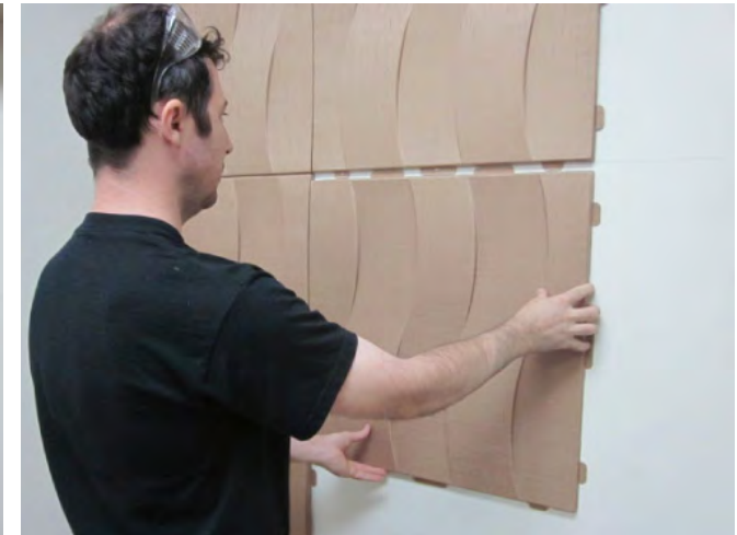
STEP 9: Continue the installation and verify the tile alignment using the reference line or laser for a symmetrical finish.
